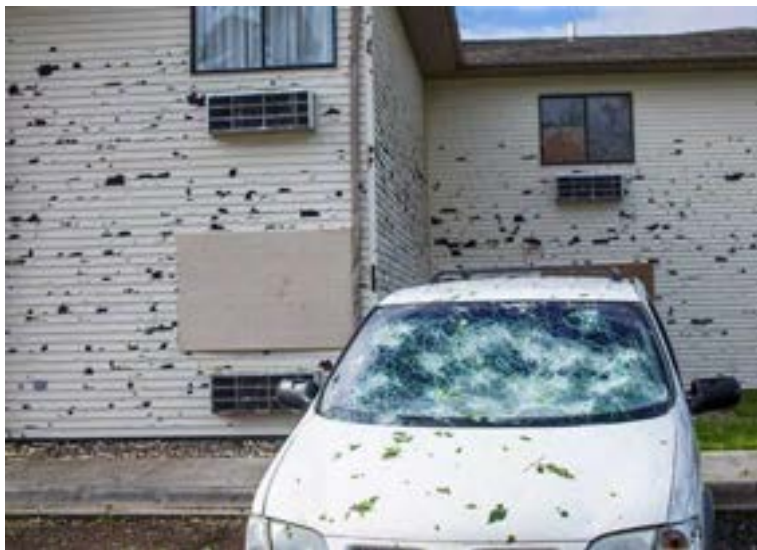
Figure 36 Damage to Vehicle and Structure Caused by Hail
