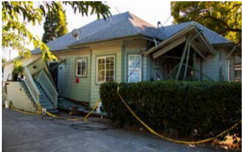
Figure 22 Structural Earthquake Damage
