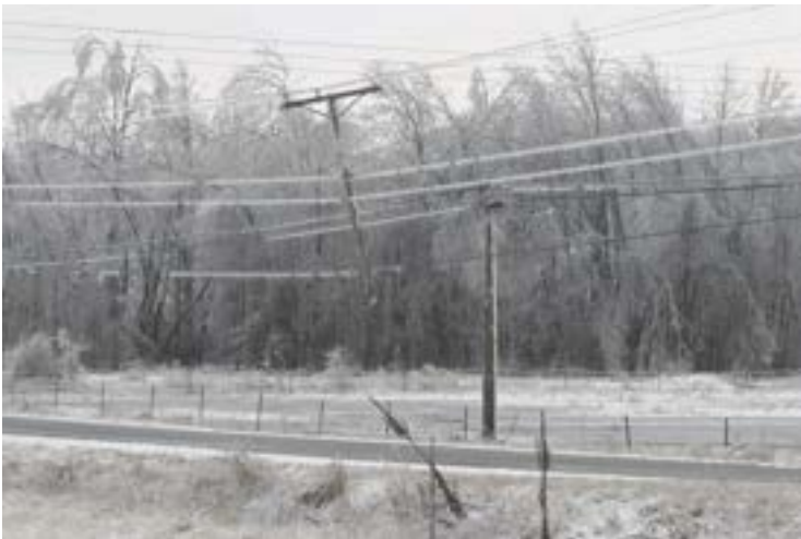
Figure 42 Ice Covered Power Lines
